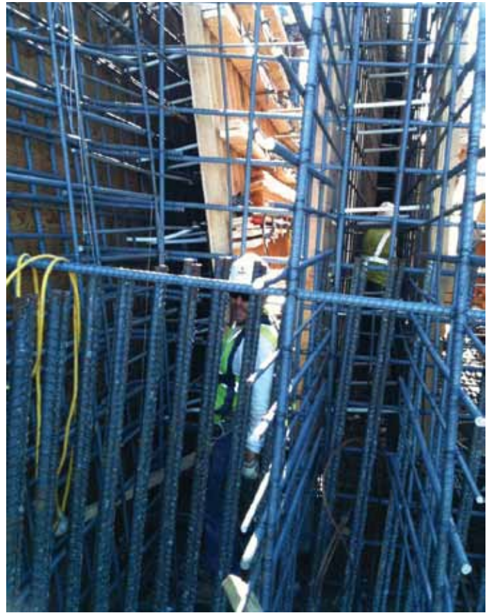
A construction worker within the tight clearances of Taxiway "R". Courtesy of Hensel Phelps Construction Co.
