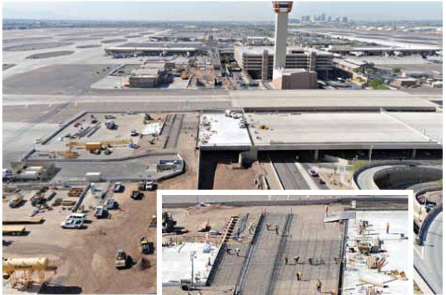
Work on the Taxiway "S" anchor slab. Courtesy of Visions in Photography.
