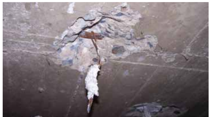
Figure 3. Corroded tie connection to steel.
