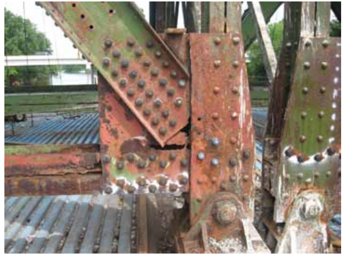
Deteriorated truss members and gusset plates prior to repair.
