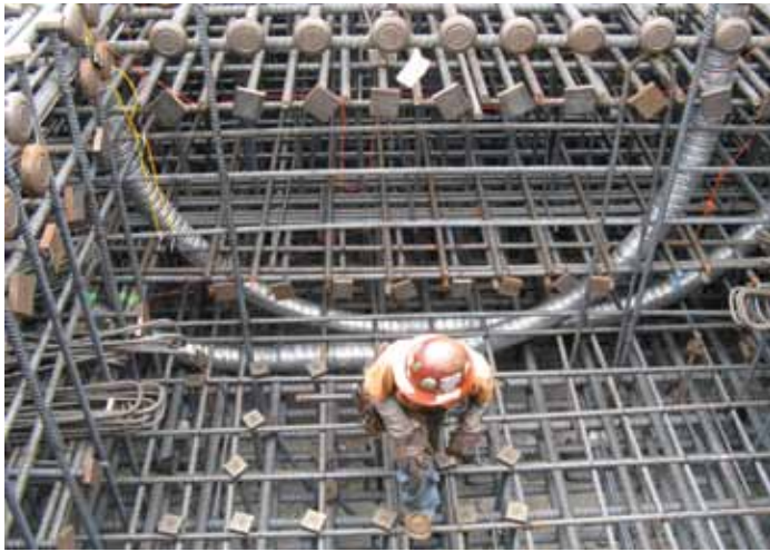
Figure 5: Mat foundation reinforcing with curved saddle for post-tensioning of the vertical post-tensioning cables.
