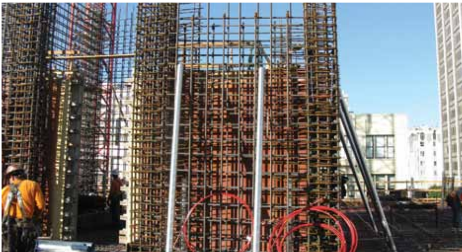
Figure 6: Core Wall reinforcing with corrugated steel ducts in walls used to post-install the vertical post-tensioning cables.
