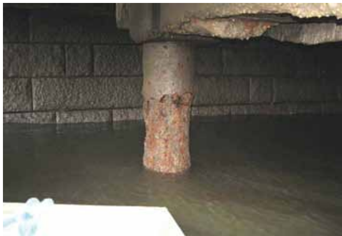
Figure 4: Corrosion of steel piles in intertidal splash zone, without protection. (Instead of showing cathodic protection, this photo shows what happens when the pile is not protected.) Courtesy of Hudson River Park Trust.
