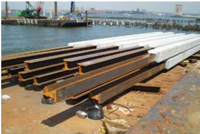
Figure 1: Hybrid steel concrete pile. The design adopted a hybrid steel and concrete pile to manage the poor soils above the rock. Courtesy of Hudson River Park Trust.
