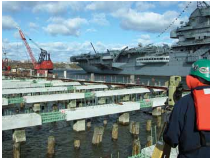
Figure 3: The installation of new concrete pile caps over the new precast concrete piles. Pile caps are elevated to avoid contact with river water. Courtesy of Hudson River Park Trust.
