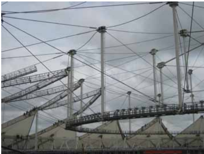
Figure 3: Interior view during construction, showing catwalk on bottom hoop cable and ridge cables at top nodes.
