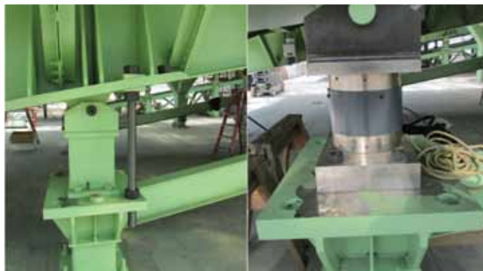
Figure 2: Jacking System (partially) and Temporary Spacer Installed (left) and Load Cell Installed (right). Courtesy of M3 Engineering and Technology.
