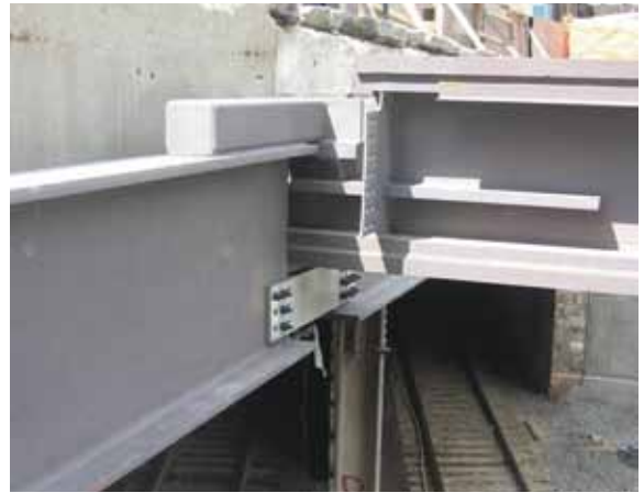
Careful detailing at the train tunnel was required to isolate members supporting the precast tunnel enclosure from the main building structure.
