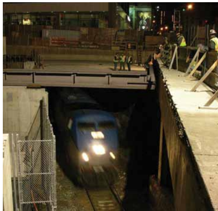
Construction over the tunnel was done at night and coordinated around the train schedule. Noise and vibration were controlled by isolating the tunnel enclosure from the tower structure.
