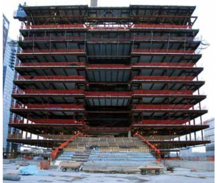
With the temporary columns removed, the load path for the hanging structure is clear. The column-free fifth floor cafeteria offers great views of the Hudson River to the west.
