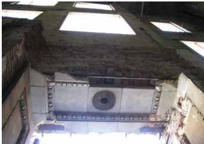
Main support beams for the façade were badly corroded. Hollow terra cotta required stabilization. Courtesy of Keast & Hood.
