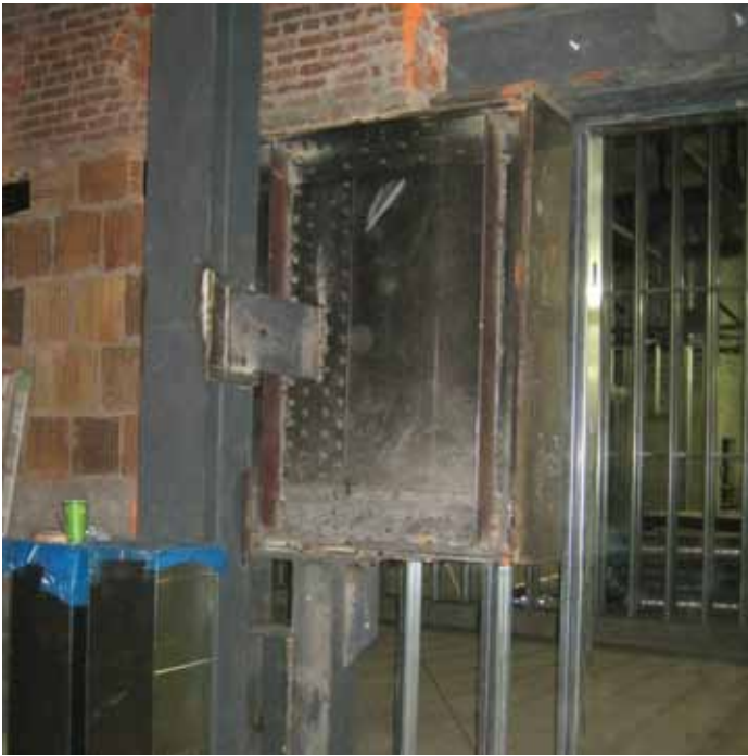
Careful sequencing ensured the proscenium alterations were done without damage to existing structure. Hydraulic jacks transferred loads until new steel structure was inserted. Courtesy of Keast & Hood.
