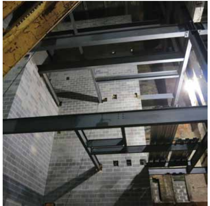
New beams fit into pockets of neoprene insulation to avoid transmitting vibration or sound through the building. Courtesy of Keast & Hood.
