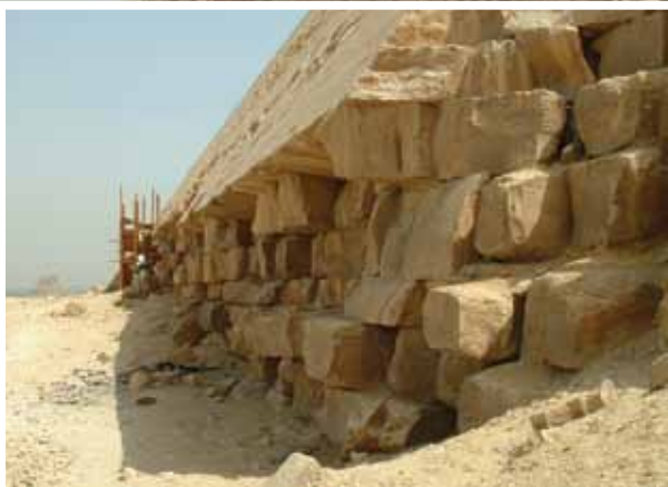
Figure 4: Limestone blocks cantilever out, where cladding below is no longer present, and eventually fail.
