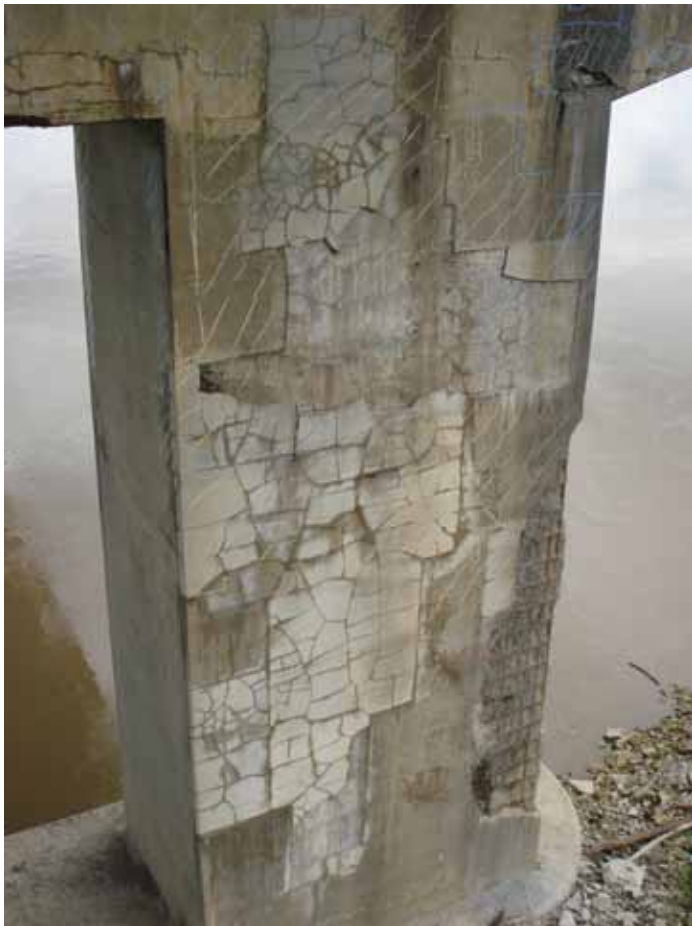
Figure 2: Pier Deterioration beneath deck joint.
