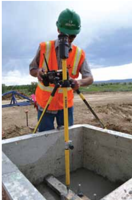
During field installation, the anchor bolt placements as well as formwork, rebar, and embeds were continuously checked using Trimble's Robotic Layout Solution – Trimble Field Link for Structures and verified in the Tekla Structures model.
