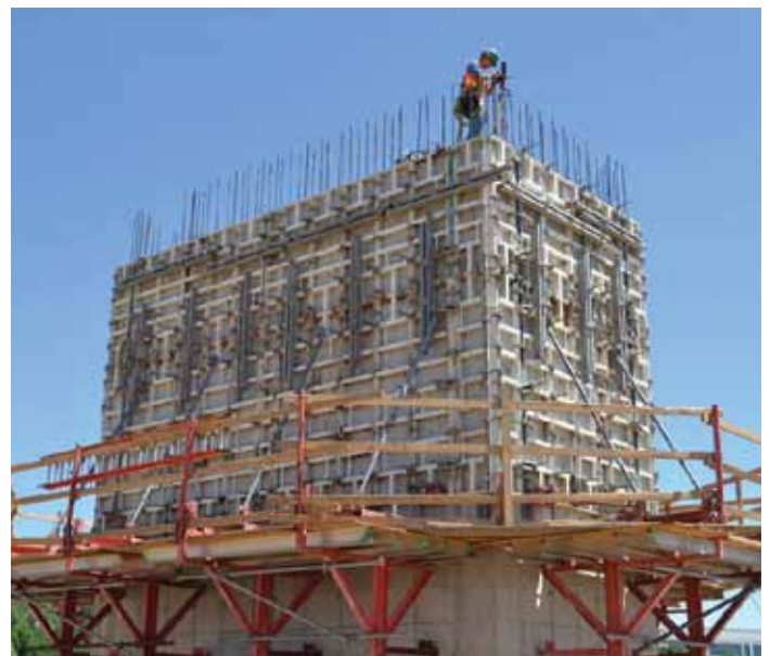
JE Dunn field personnel using the Trimble RTS 773 and Trimble Field Link for Structures layout solution for verifying edge of slab during the build-out of the elevator core.
