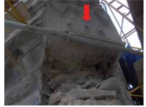
Figure 9b: Partial buttress removal below the the pinned stones in Figure 9a.
