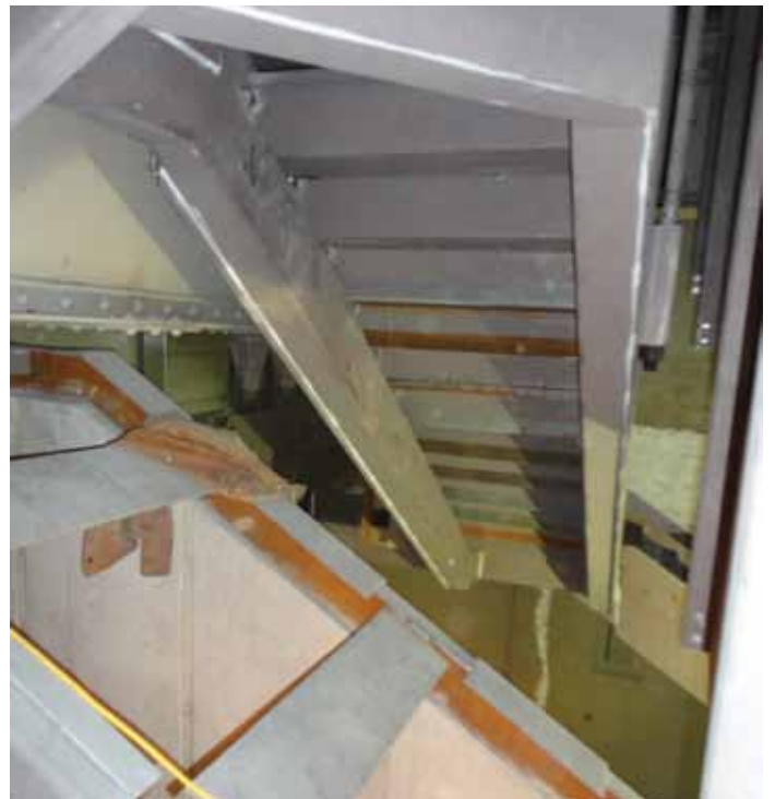
Tight clearances for new steel at the existing Eiffel girders. Courtesy of Keast & Hood Co.
