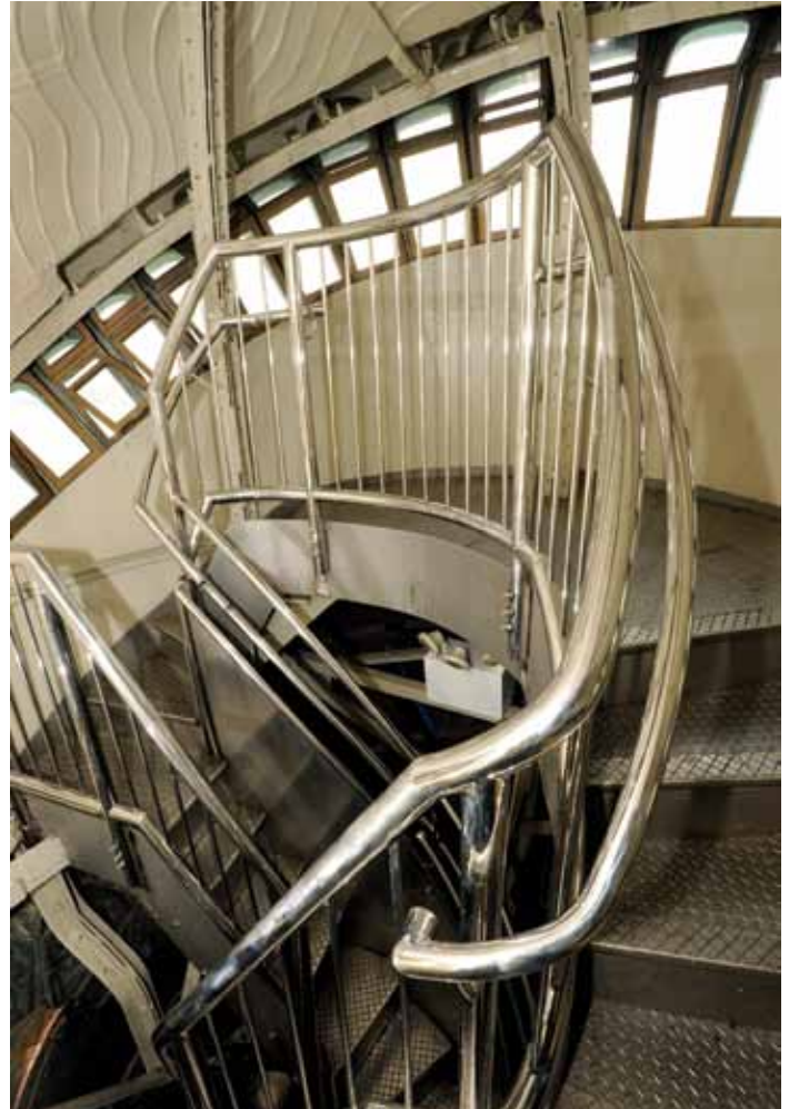
New handrail in the crown at the top of the spiral stairs. Courtesy of National Park Service.
