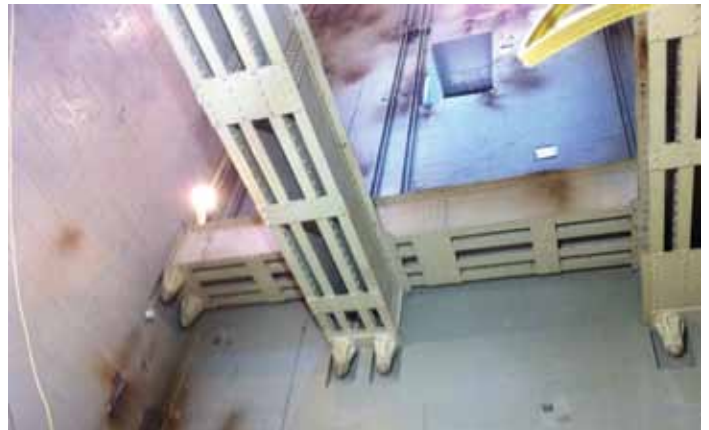
View of pedestal interior above level 3P after demolition. Courtesy of Keast & Hood Co.
