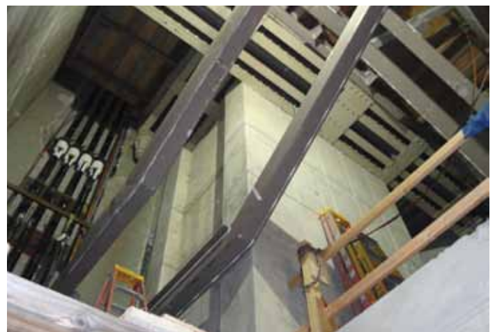
New elevator shaft and stair framing above level 3P. Courtesy of Keast & Hood Co.
