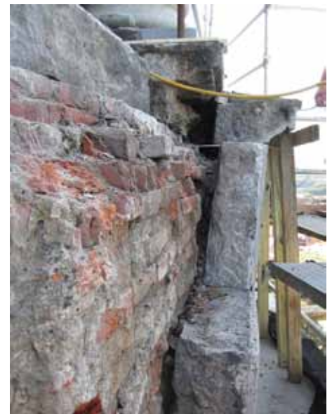
Figure 7: Deteriorated masonry behind granite ashlar cladding at exterior of lower drum.
