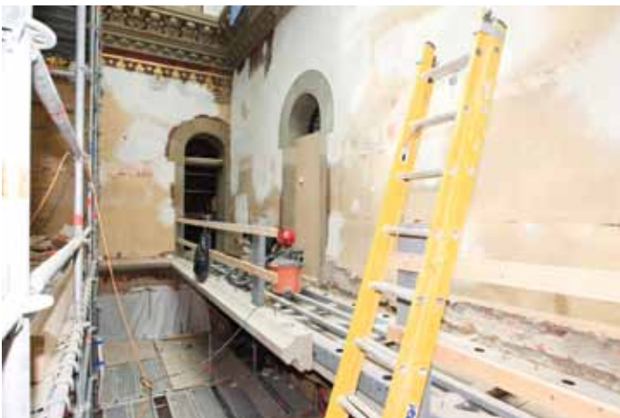
Figure 6: Balcony steel frame and sandstone cladding installation during construction. Courtesy of Laurie Donald, Bernstein Associates Photographers, for OGS.
