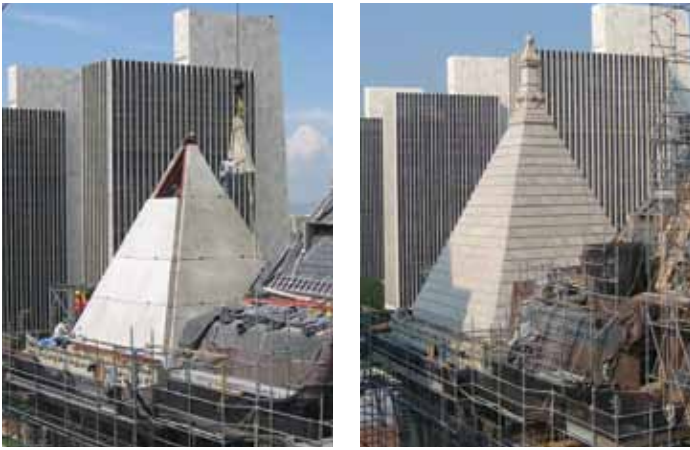
Figure 3: Granite tower during installation of new substructure and after reinstallation of granite.
