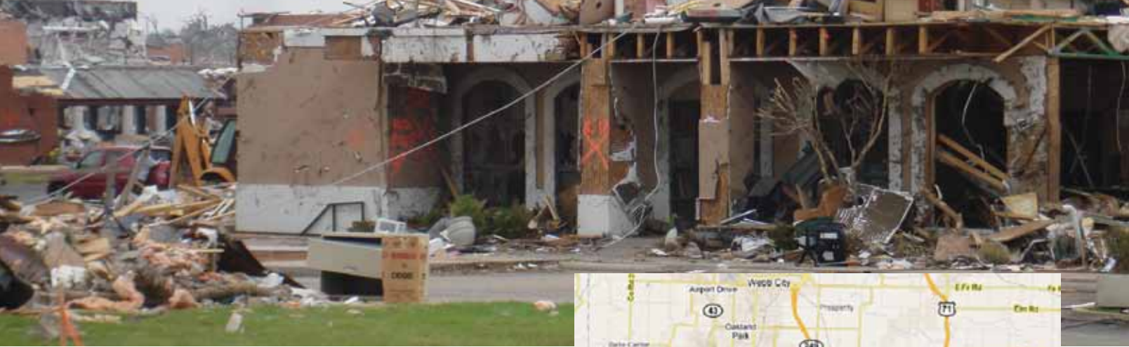
Non-residential building remains standing despite major damage.
