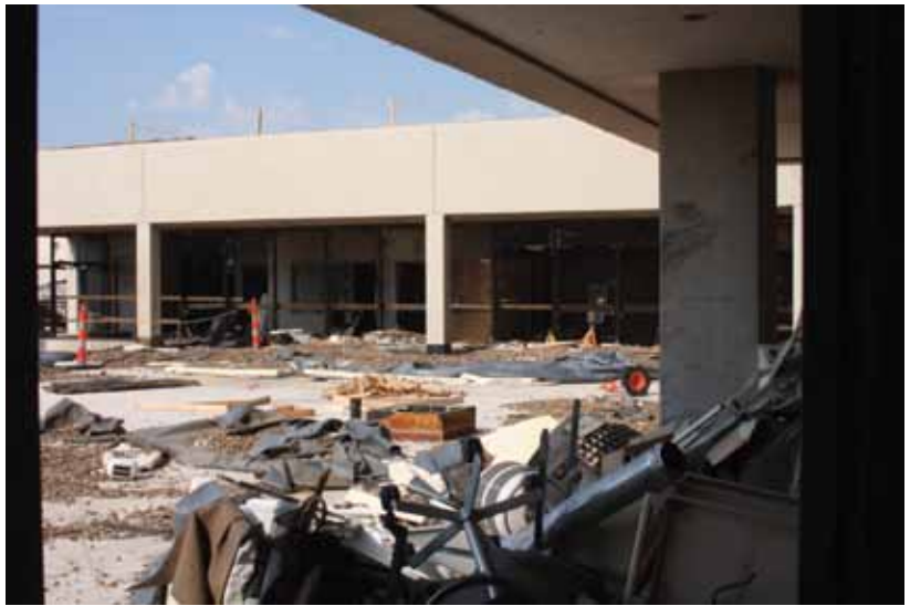
St. John’s Hospital damage; note the ballasted roof, lightweight concrete and glazed curtain wall destruction.
