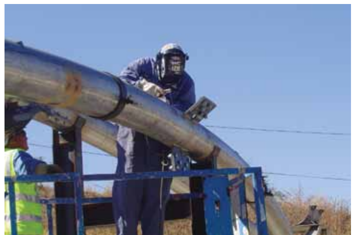
Temporary plates, braces, and supports help to fit up the mid-span weld of the crossed arches pipe bridge.
