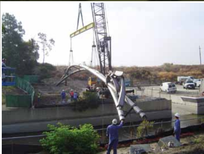
American 7150 Mobile Crane hoists completely assembled crossed arches pipe bridge into position.
