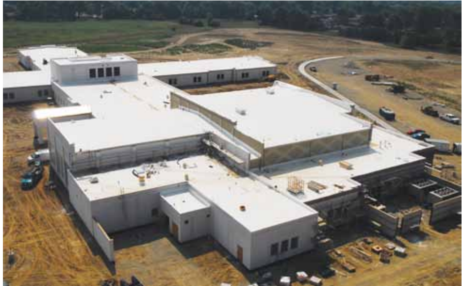
Trotwood Middle School, Trotwood Ohio employed an AAC structural wall system comprising prefab steel reinforced AAC wall panels and AAC masonry block load bearing walls.
