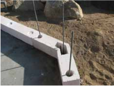
Private residence construction showing a block base course and bored cores with vertical steel reinforcement. Cores will be grouted for structural continuity across block.
