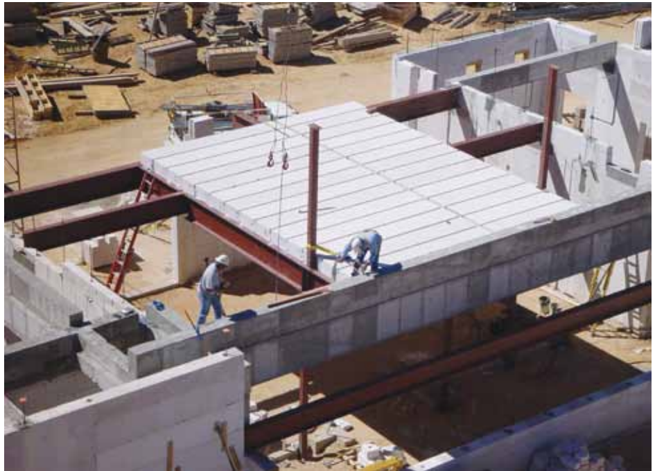
Sky Indian Cultural Center at Acoma Pueblo, New Mexico employed AAC structural building systems throughout, including AAC masonry block, prefab vertical reinforced panels and prefab reinforced floor panels.
