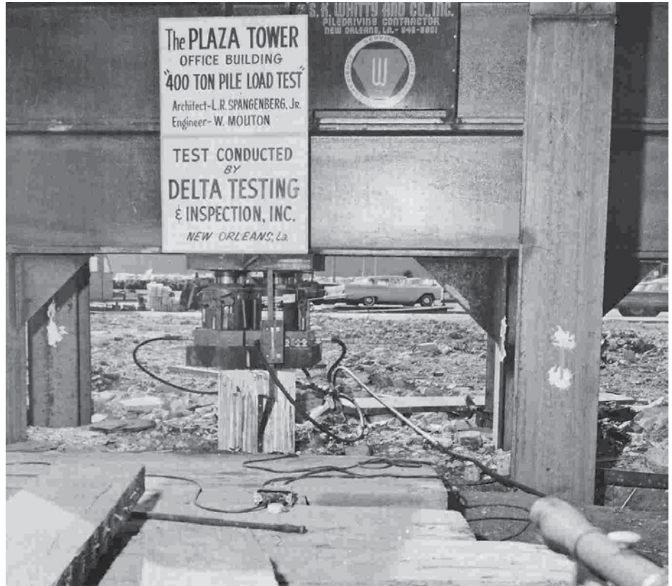
Figure 3: Pile testing for the Plaza Tower was pushed all the way to 462 tons without failure, well in excess of the required 180-ton design load. Courtesy of Mary Mouton.
