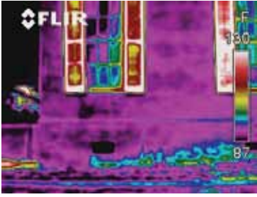
Figure 4: Infrared thermography image showing areas of rising damp and path of moisture travel.
