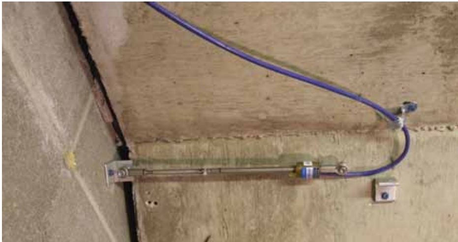
Figure 6: Vibrating wire crack monitors used for long-term structural movement monitoring.
