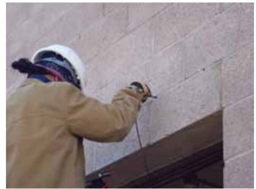
Figure 1: Using a fiber optic borescope inserted into a drilled hole in a mortar joint to view the inside of a concrete masonry lintel.
