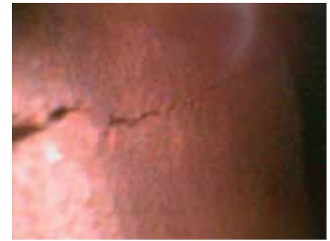
Figure 8: Borescope image of a crack forming on the back face of a veneer panel.
