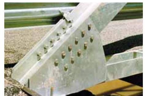
Hot-dip galvanized bolts used on connection of structural members.
