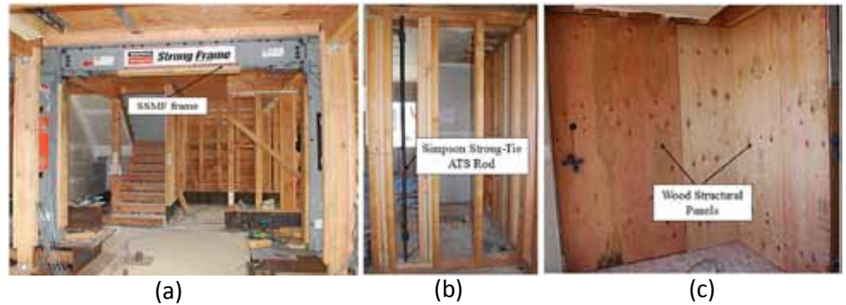
Figure 5. (a) East span of Strong Frame installed parallel to the motion of shake table. (b) ATS rods and stud pack inside wood shearwall. (c) Plywood panels at upper stories.
