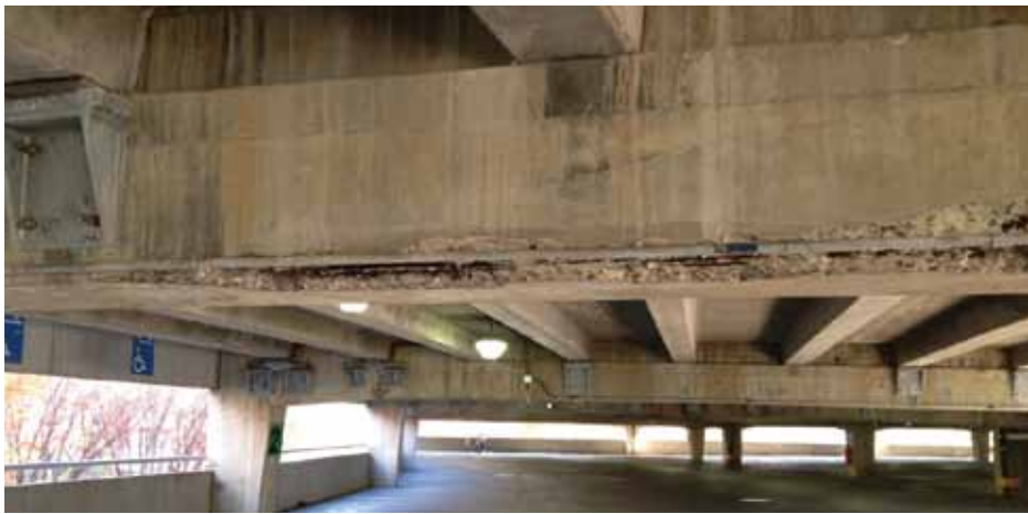
Figure 2: Spalling due to deteriorated strands at precast girder.
