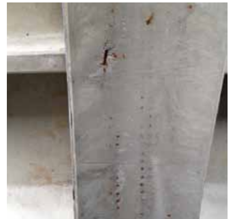
Figure 4: Rust staining due to internal corrosion of post-tensioned girder reinforcing.
