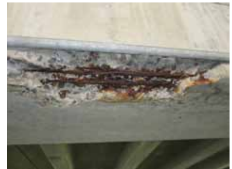
Figure 3: Corroded and failed prestressing strands at precast girder.
