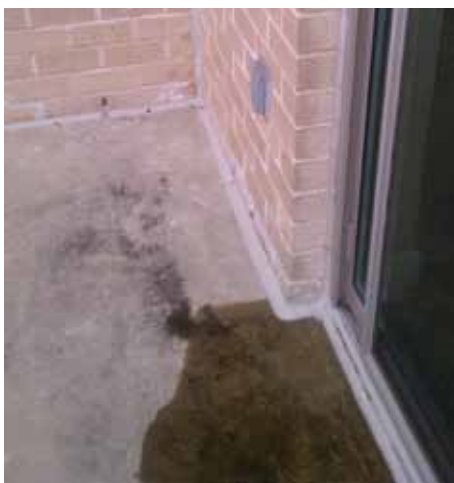
Figure 9: Water ponding at an existing balcony.
