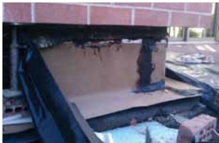
Figure 10: Typical completed through wall flashing repair for remedial fix to balcony drainage issue.
