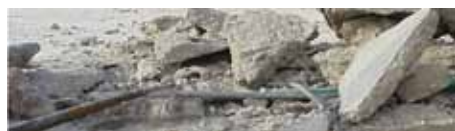
Figure 5: Crushed PT ends at a balcony slab edge.
