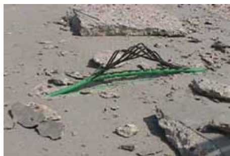
Figure 6: Tendon popout at a balcony slab.
