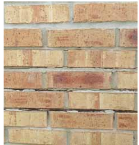
Figure 3. Fence breaking apart from corrosion of joint reinforcing. Fence was less than 2 years old at time of photograph in 2005, Austin, TX.
