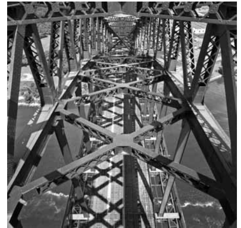
Inside Hell Gate Truss arch, looking down onto the tracks. The truss is 53 feet wide over 4 tracks. Note the lateral bracing and the heaviness of the structural materials. The sidewalks flanking the tracks are capable of supporting an overhead trolley. Courtesy of Dave Frieder.com. All Rights Reserved.
