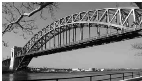
The Hell Gate Bridge today: The truss arch members structure highlighted under sunlight. Courtesy of Adam J. Kirk 2011.
