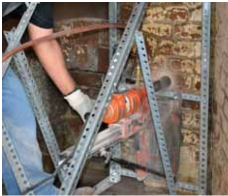
Figure 2: Coring of material samples revealed that although the construction drawings indicate a brick wall across the width, the construction of the fort is composite with tabby concrete infill.
