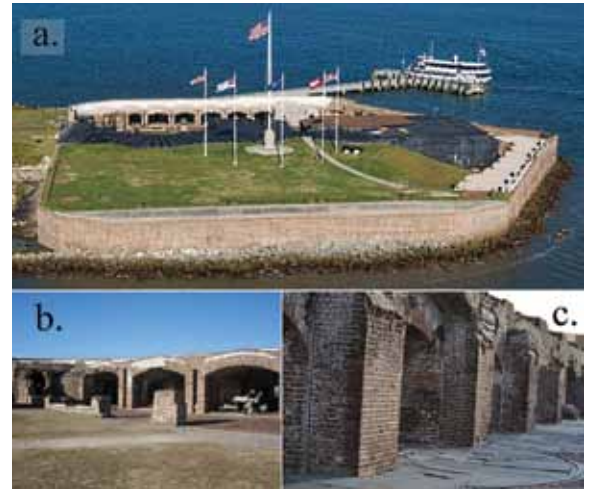
Figure 1: The current state of Fort Sumter National Monument: (a) aerial view, (b) barrel vaulted casemates, and (c) degradation of brick and mortar piers.
