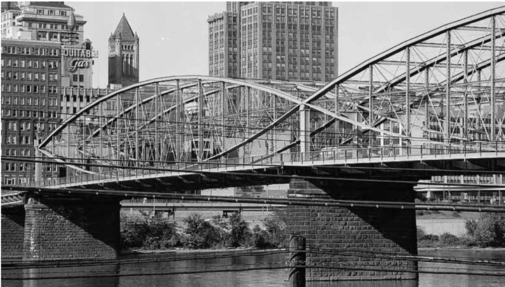
The superb lenticular spans and wide piers, seen from the west. It is the oldest and longest through-truss extant bridge in the U.S. HAER PA-Pitbu, 58-9. Jack. E. Boucher, Photographer. 1974.
