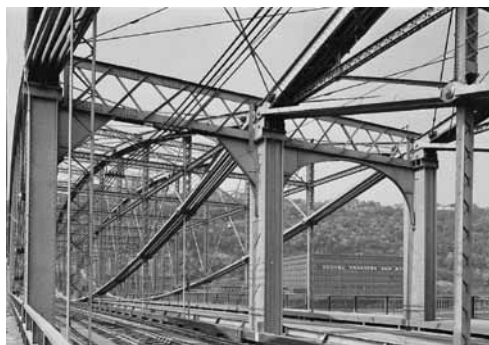
Interior through-truss with the third set of lenticular trusses of 1891 (left) first for horse-drawn trolleys, later for the 1898 electric trolley track. Lindenthal extended the bridge's service life via planned, sustainable design. HAER, PA-2 Pitbu, 58-18. Jack E. Boucher, 1974.
