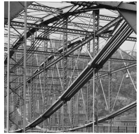
Close up of steel plate top and bottom chords, acting as arch and cable. The wrought iron vertical members are seen, with the horizontal intermediate bracing at midpoint running the length of the bridge. HAER, PA-2 Pitbu, 58-18. Jack E. Boucher, 1974.
