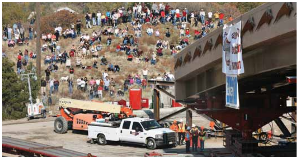
Use of accelerated construction techniques on a Utah bridge project attracted local spectators and highway professionals from across the country.
