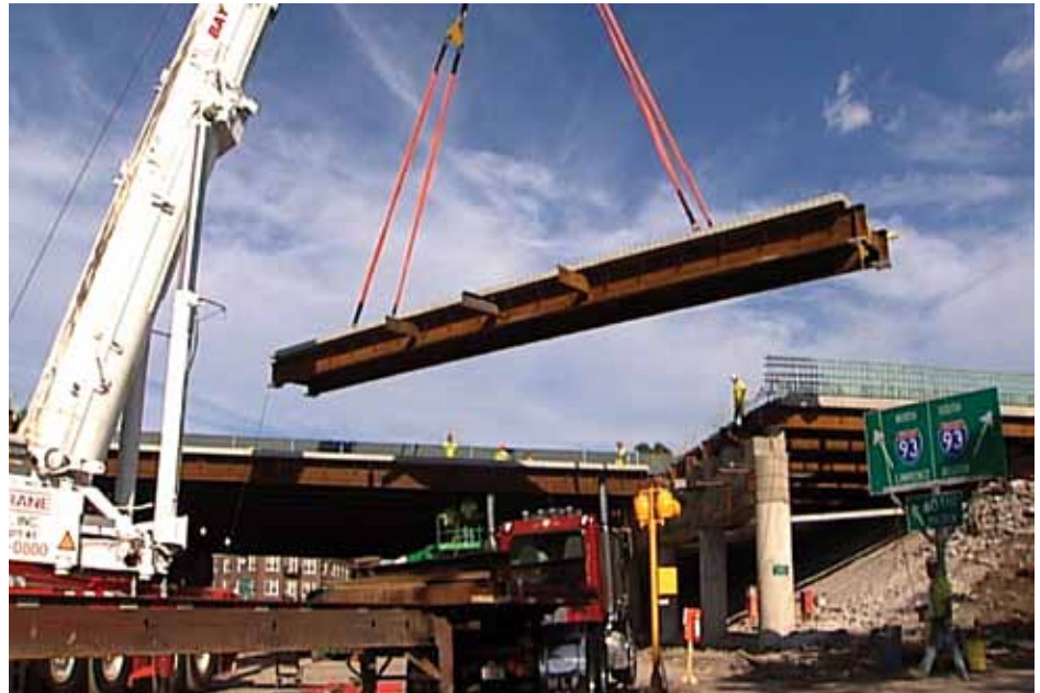
Workers used ABC techniques to replace 14 Massachusetts bridges in one summer while minimizing impact on drivers.
