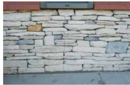
In any good masonry design, one must account for movement of the veneer and the backing. Cracks resulting from movement are unsightly and can be both difficult and expensive to repair.
