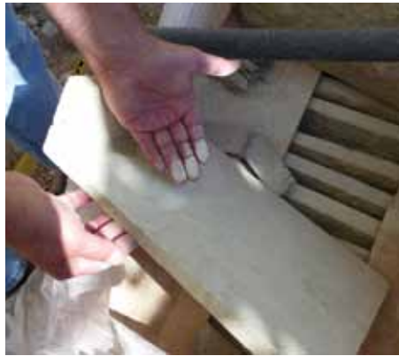
Material may require a thorough cleaning to ensure adequate bond between the veneer and backing.
