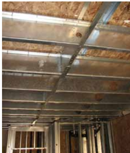
Figure 3: Blocked wood sheathed CFS framed diaphragm. Courtesy of Don Allen of DSi Engineering.
