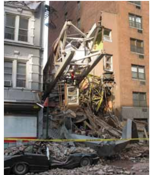
Figure 1: On the Upper East Side of Manhattan, a tower crane collapsed during a climbing operation, resulting in multiple deaths and massive property damage.
