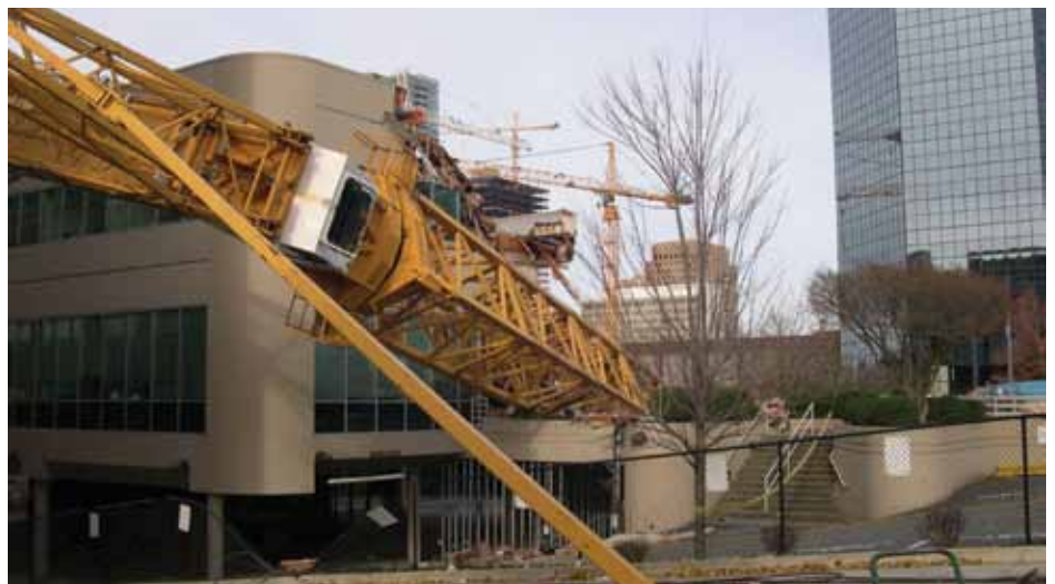
Figure 5: A tower crane toppled after its base frame failed.
