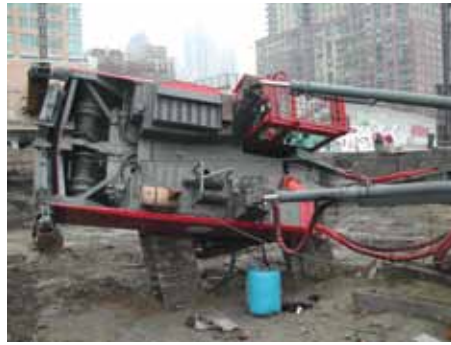
Figure 3: A crawler crane relies on firm level ground support to keep it from tipping.
