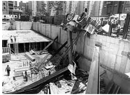
Figure 4: Telescopic crane toppled into a construction site, pinning a passerby.
