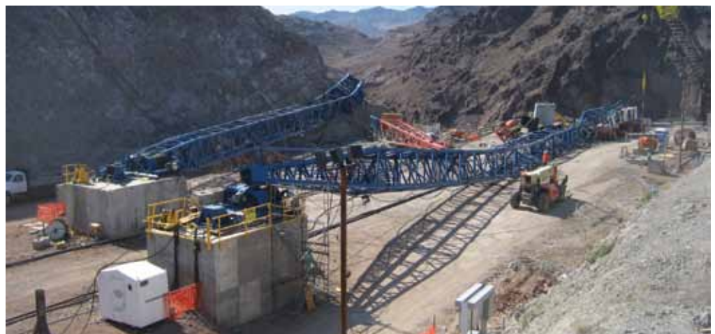
Figure 2: A half-mile-long cableway across Black Canyon on the Colorado River collapsed during high winds. Its loss set back construction of a vital interstate bridge link by two years.
