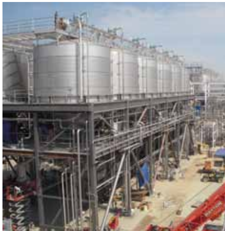
The new Special Concentrically Braced Frame (SCBF) structure at the winery, configured to support massive fermentation tanks at their second story.
