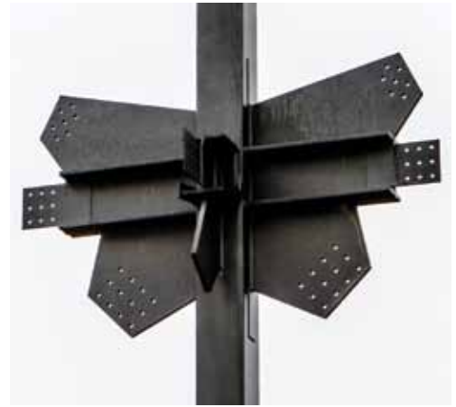
“Butterfly” gusset plate connection. The gusset plate is continuous through the column to accommodate the significant pass-through forces imparted to the braces during an earthquake; beams and braces are field-bolted to the column.
