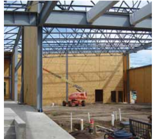
SIP wall panels go up first, followed by the roof panels, providing a strong, well-insulated building enclosure.
