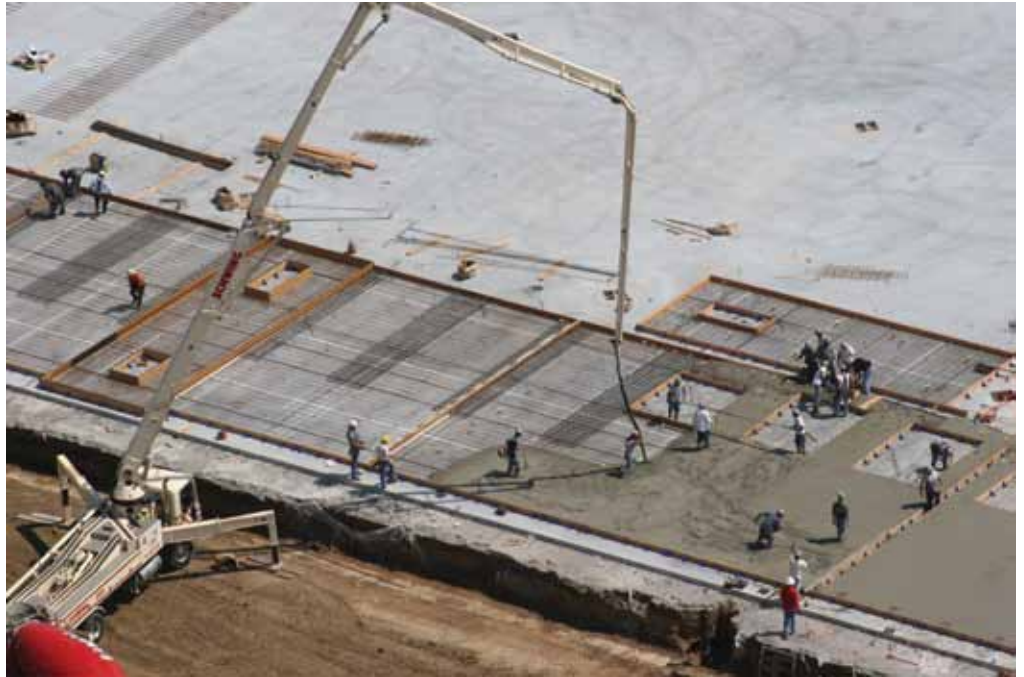
These panels were reinforced using a single uniform mat of WWR throughout, with tied rebar cages (two mats of rebar) added at jamb strips. Courtesy of Lithko Contracting, Inc.
