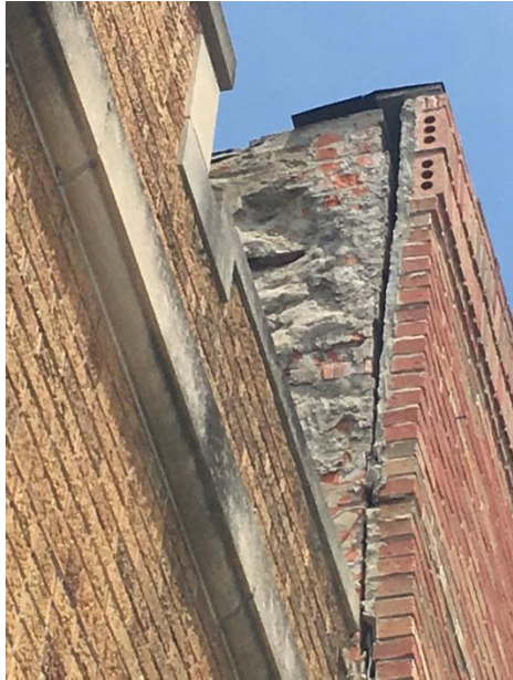
There could be no existing wall ties
