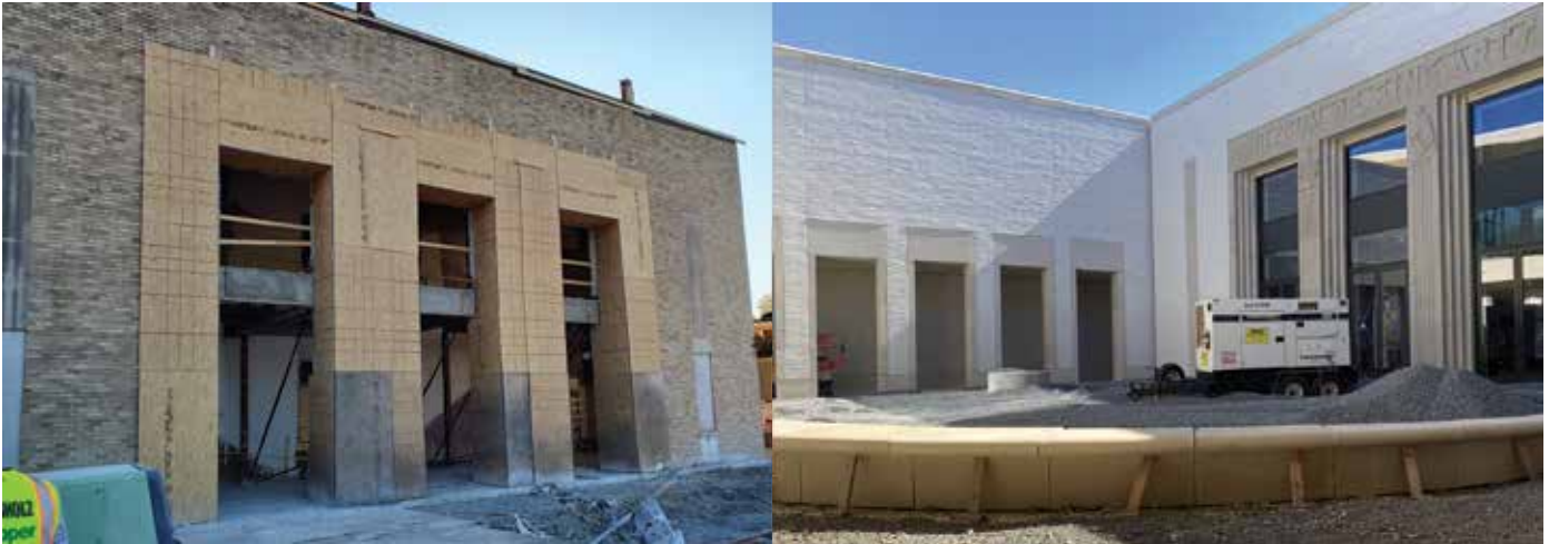
On the left, protection was required to preserve the limestone of the original Museum of Fine Arts. On the right is the restored façade, including the replaced exterior wythe of brick. Courtesy of Polk Stanley Wilcox.
