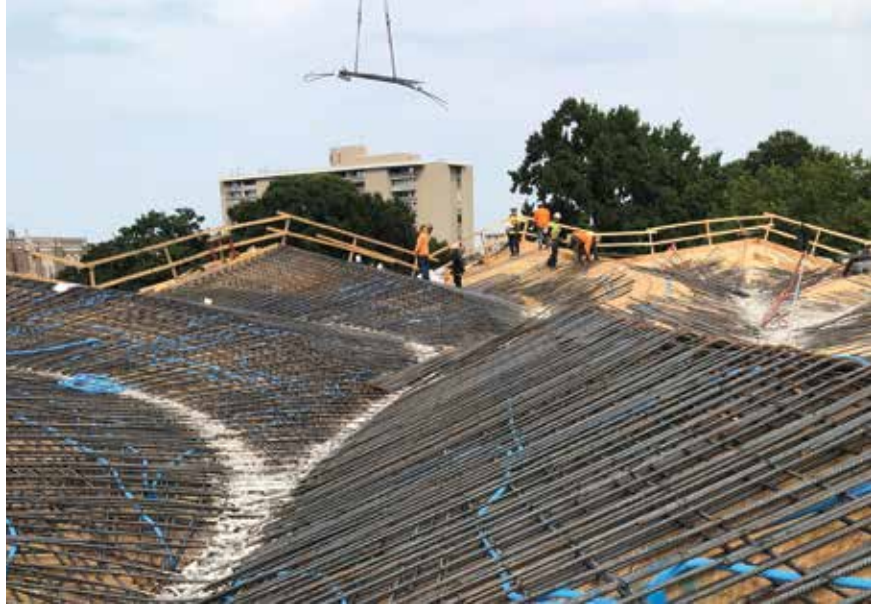
Rebar placement on the Courtyard Entrance roof. Courtesy of Polk Stanley Wilcox.
