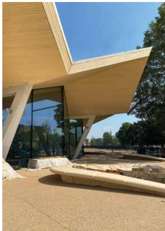
The Park Entrance roof nearing completion with site work in progress. Courtesy of Polk Stanley Wilcox.
