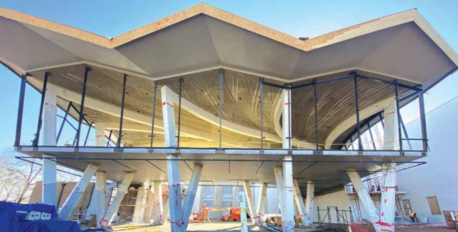
The reimagined Arkansas Museum of Fine Arts and its folded concrete roof. Courtesy of Polk Stanley Wilcox.
