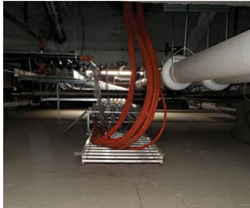
Figure 1. Various utilities go in and out of data center facilities into a crawl space of a seismically isolated building.
