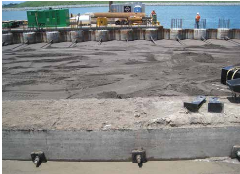
Lightweight fill placed between the A-frame pile cap and the combi-wall. Courtesy of Gary Ledford.
