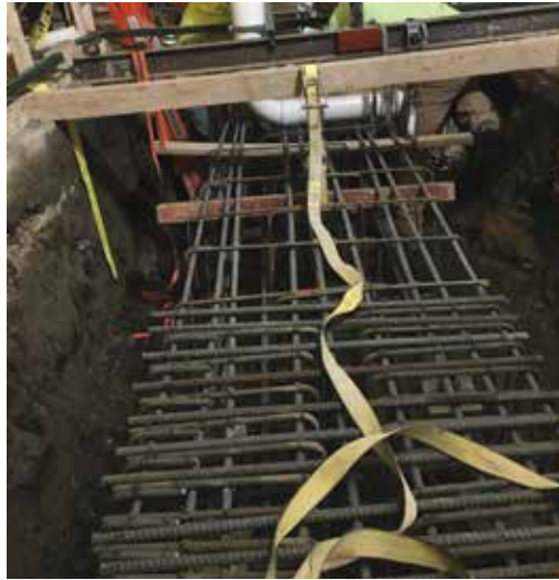
Figure 7. Grade beam reinforcement placed around the tops of micropiles, adjacent to existing stair.
