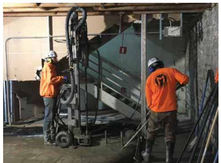
Figure 6. Micropiles being installed through the basement slab adjacent to the existing stair.
