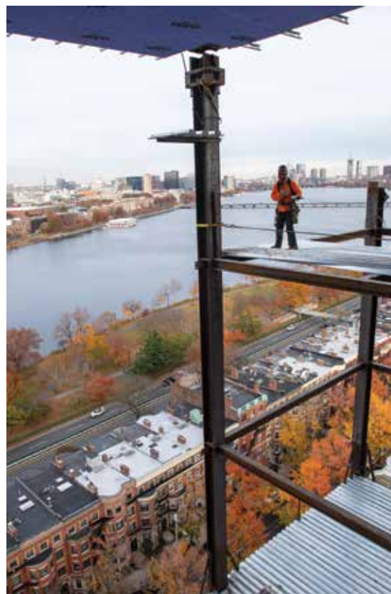
Temporary shoring removal after unloading. Courtesy of Cydney Scott, Boston University Photography.
