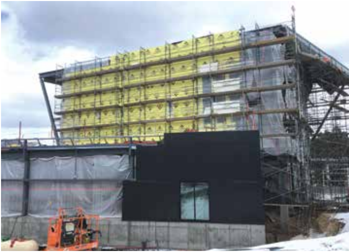
Figure 5. The structural team coordinated multiple systems and unique deflections while maintaining a cohesive design.
