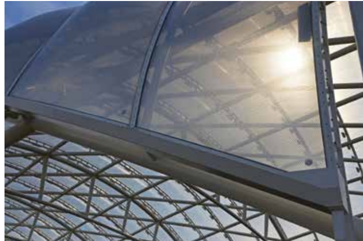
Ethylene tetrafluoroethylene allows for abundant natural light, reducing lighting and energy costs during operation. Courtesy of Nigel Marson Photography.
