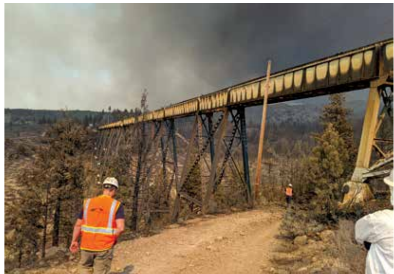
View of the west side of the damaged bridge looking north from the south embankment.
