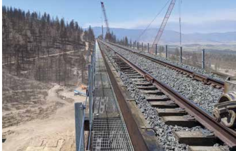
View of the completed bridge deck looking south from the north abutment.
