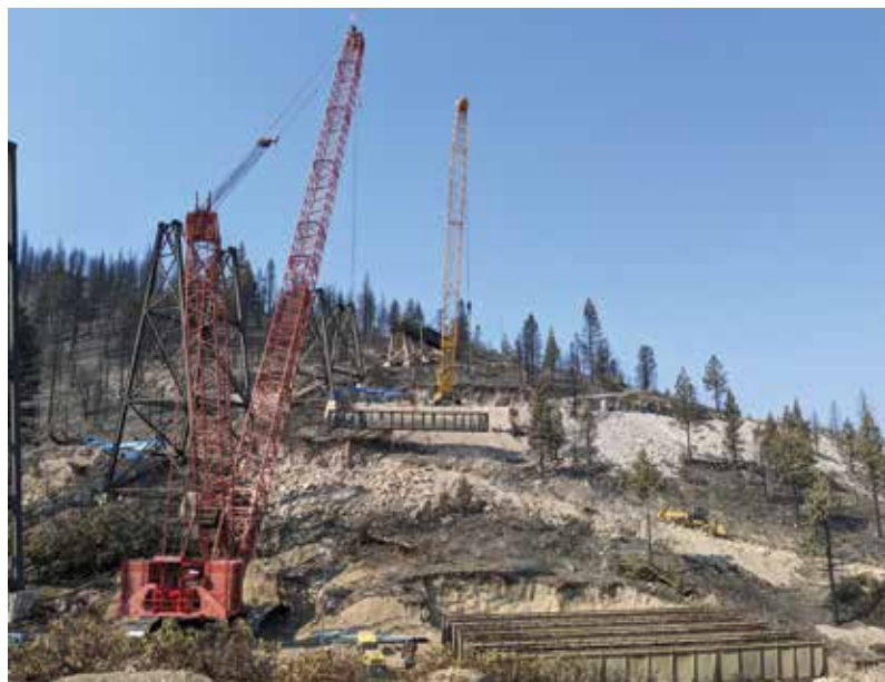
View of the removal of Span 3. Crane positioned alongside the south embankment passing the span to another crane downhill.
