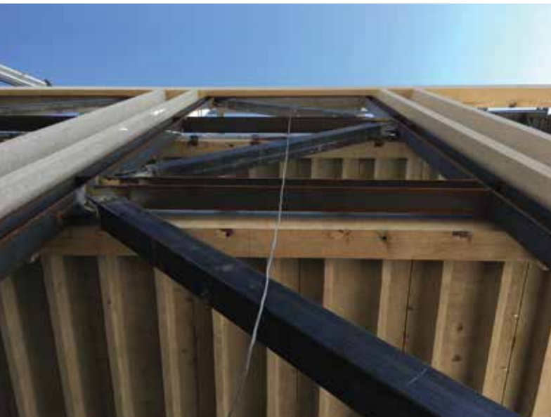
Figure 2. A new BRBF was installed in-plane with the pre-cast concrete columns and outboard of the floor girders.
