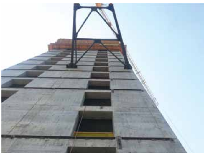
Figure 2. The coupled shear wall core of a multistory building in the Seattle area. Courtesy of Cary Kopczynski & Co., Bellevue, WA.
