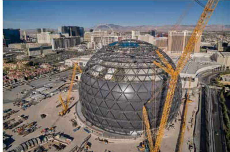
The MSG Sphere at the Venetian's exosphere is the largest spherical structure on Earth, was parametrically designed and optimized by Severud Associates, and features cast steel nodes by CAST CONNEX. Courtesy of Mike McNulty.
