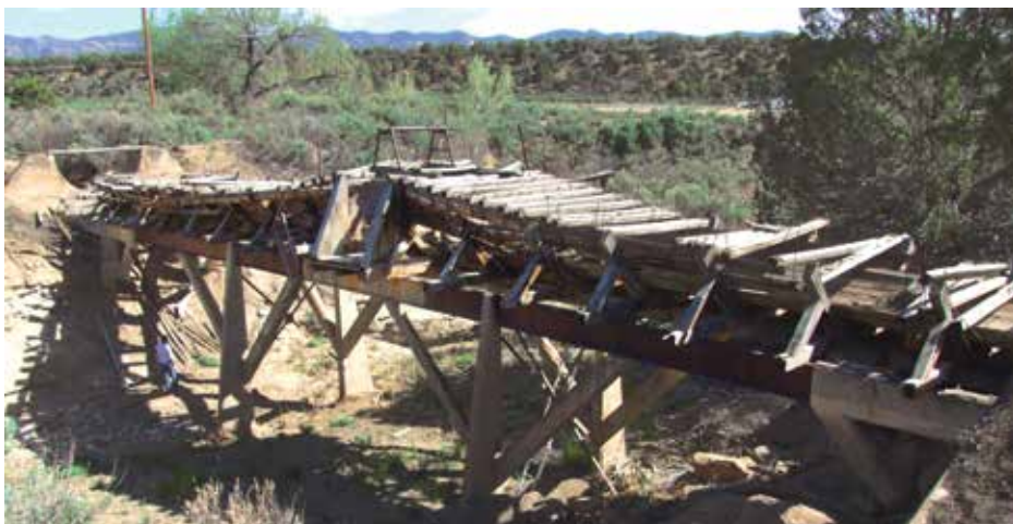
Figure 2. The McElmo Flume in 2012 in a state of partial collapse due to damage from severe natural events.
